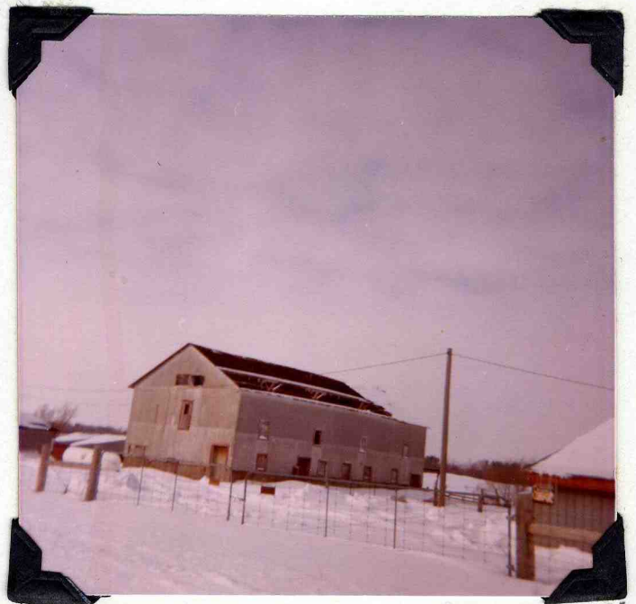
Ralph Gooding's barn 10th conc. Roof damaged
