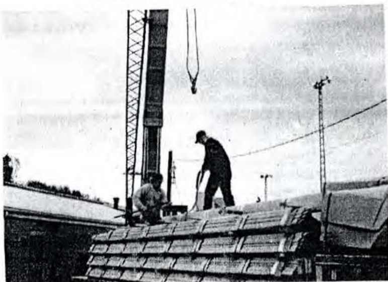
The new roof was started last week at the West Elgin Arena. Here they are unloading the roofing material. It won't take long if the weather co-operates with the workers. OCT 98
