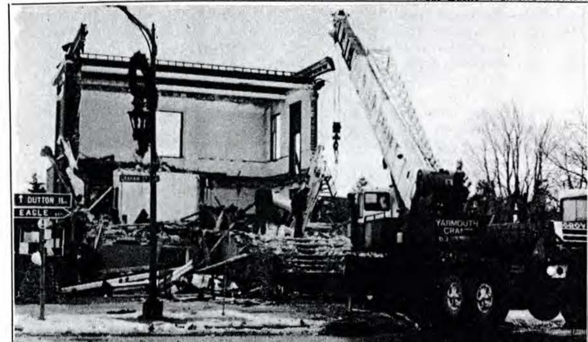
Going Going Gone... The Old West Lorne Community Hall came tumbling down last week but not before this heavy construction vehicle was uprighted after falling through the ground floor into the basement of the old hall. Photo by Brian Outhouse.
