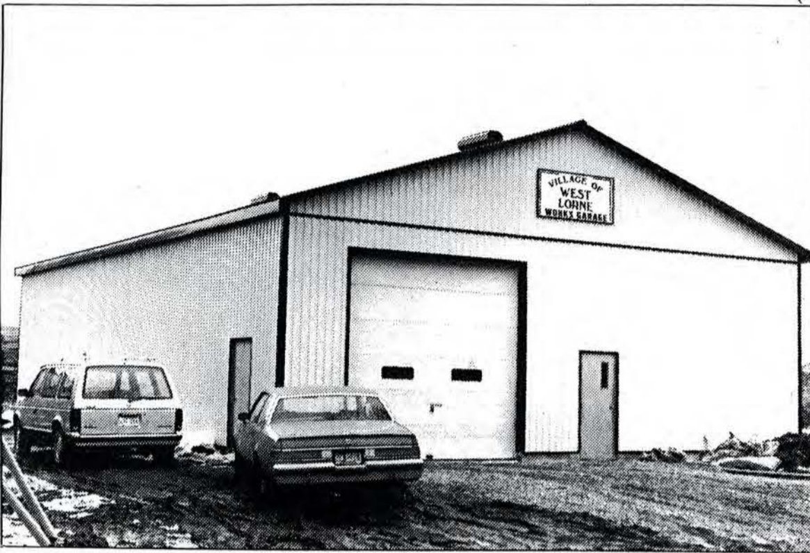
WORK PROGRESSES ON NEW WORKS GARAGE -- The new West Lorne works garage which will soon be used by town employee George Nute to house the town's vehicles and equipment. (Photo By Brian Outhouse)
