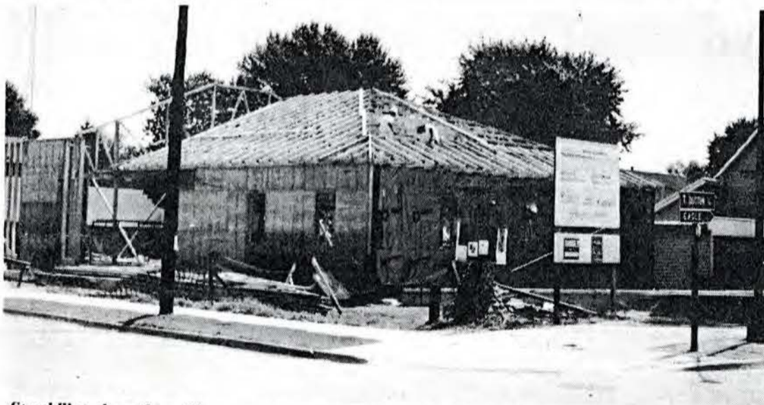
Straddling the rafters- These construction workers for Van - Ver Construction are seen installing the framework for the roof of the new Town Hall in West Lorne recently. Construction of the final phase of the Community Complex has been moving along on schedule according to the builders of the new structure. (Photo by Brian Outhouse).
