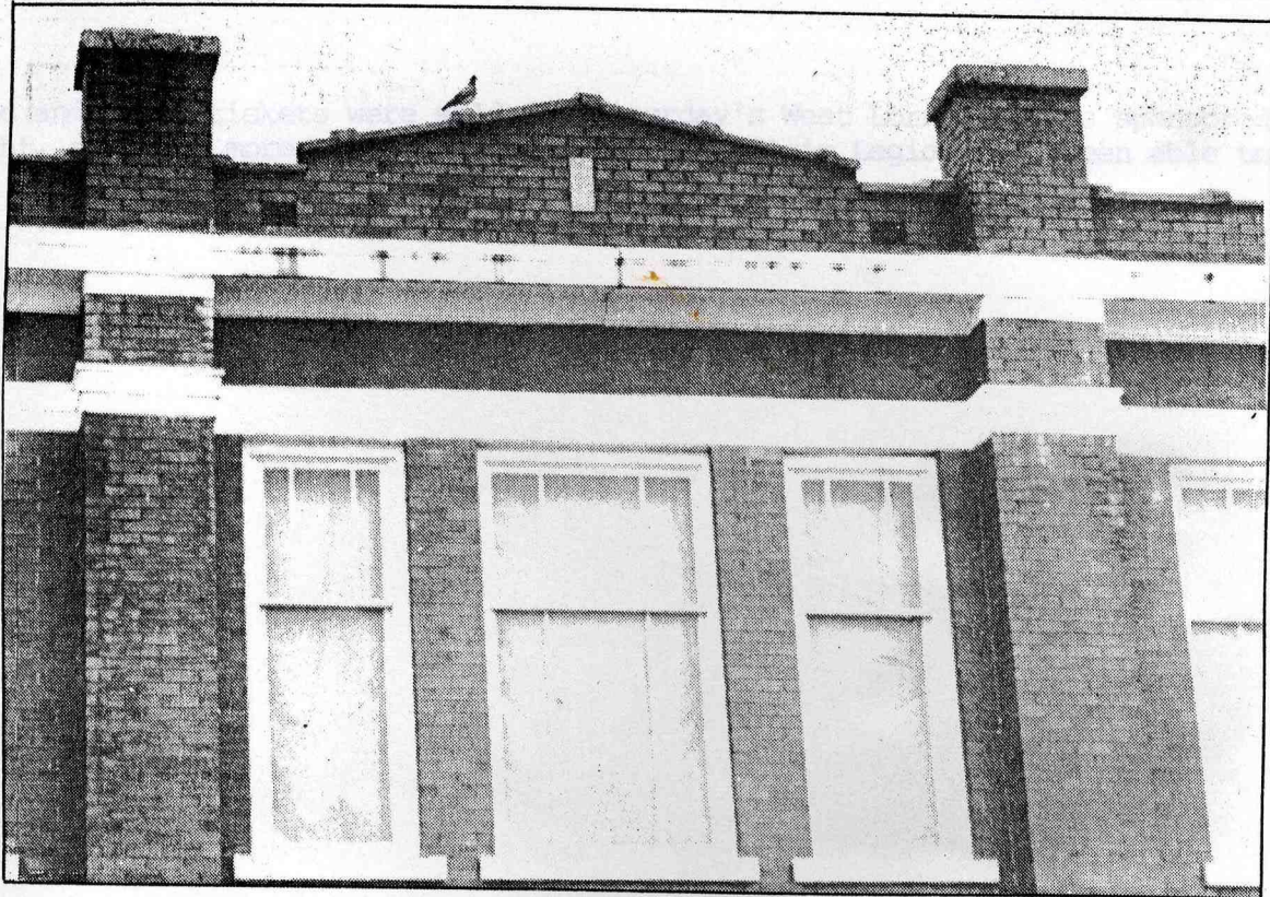
This pigeon makes its home in an air vent in West Lorne's town hall. The roof leaks and chimney bricks are practically falling off. Wheelchair ramps must be installed next year.
