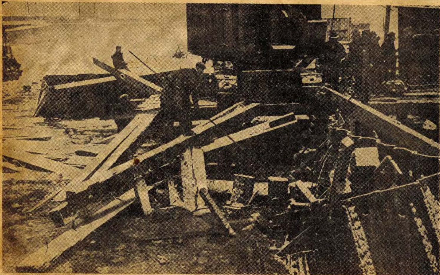
Workers are seen in the above view of the wrecked coffer dam at Port Stanley endeavoring to dislodge with pike poles timbers jammed in the hole that had been the coffer and in which at the time the photograph was taken, eight men were still entrapped. The picture was
