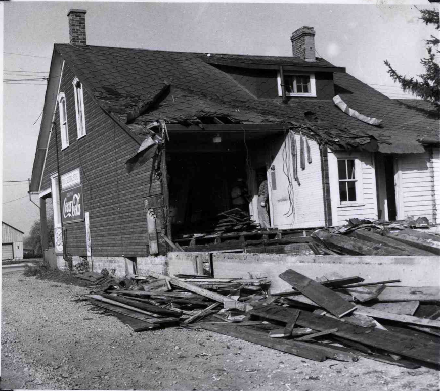
The Yarmouth Centre General store, for more than 80 years a landmark of Yarmouth Township, is being torn down by the Department of Highways to provide a clear view of the intersection of Highway No 3, and the sideroad. Oct. 1963.
