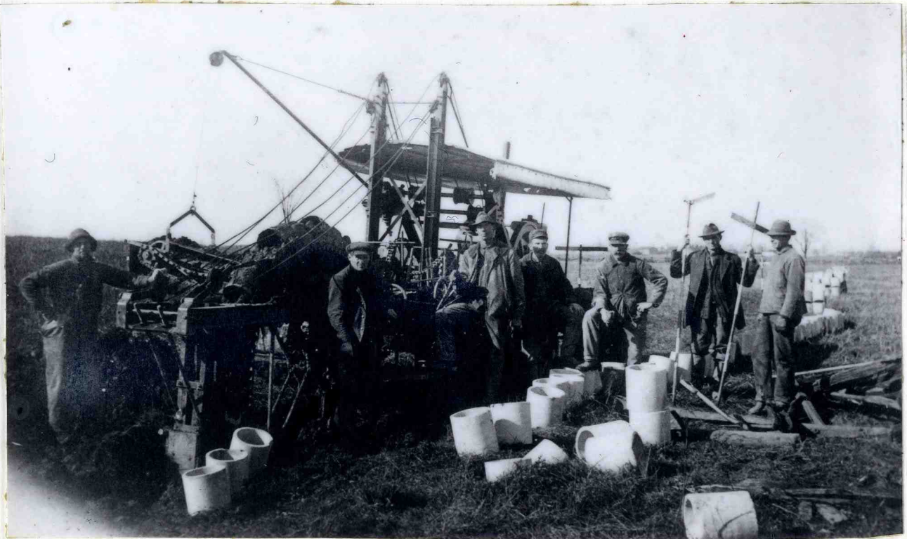
This ditching machine for laying drainage tile was owned and operated by James Reid.
